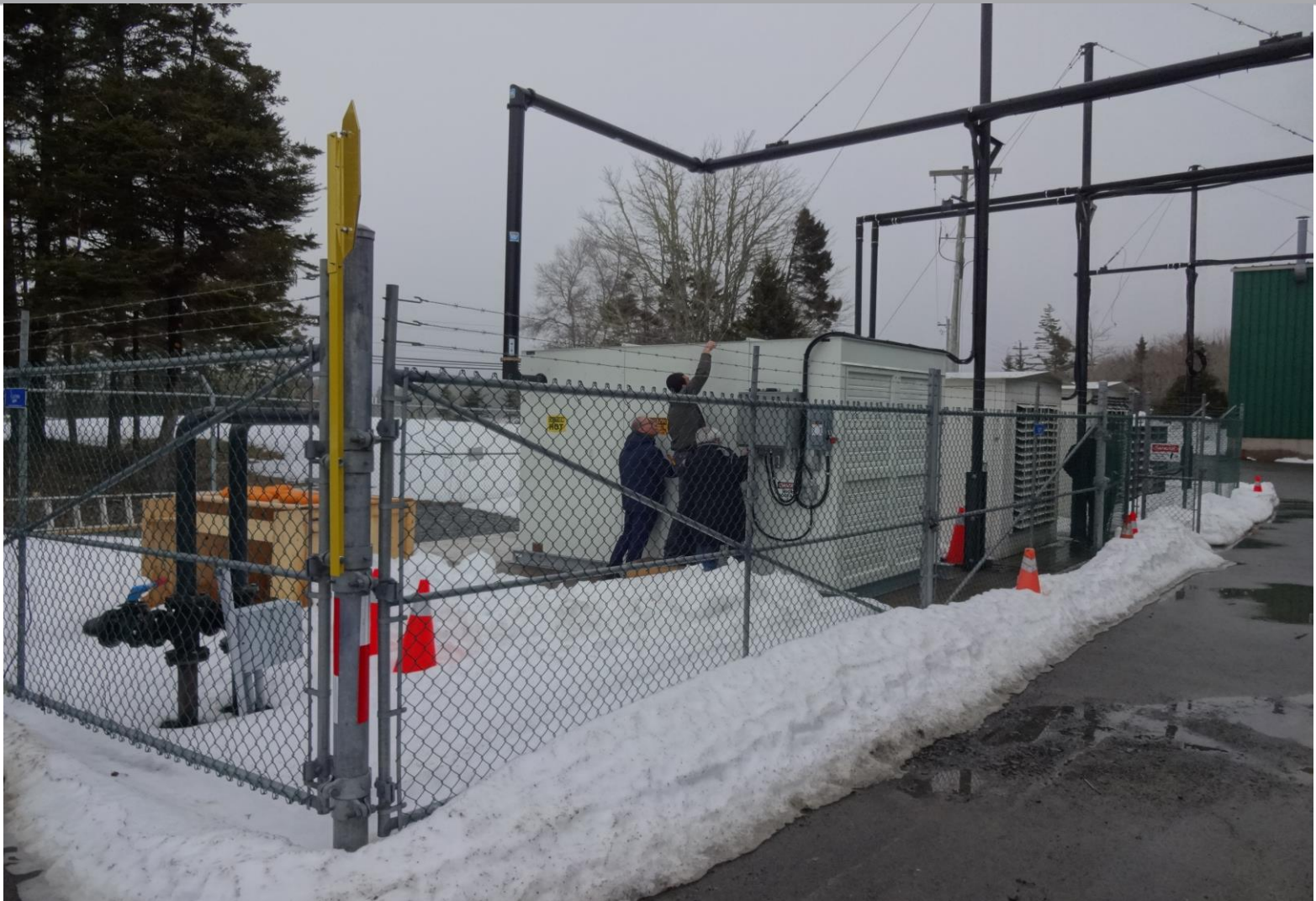
Nautel installs a new 400kW load
